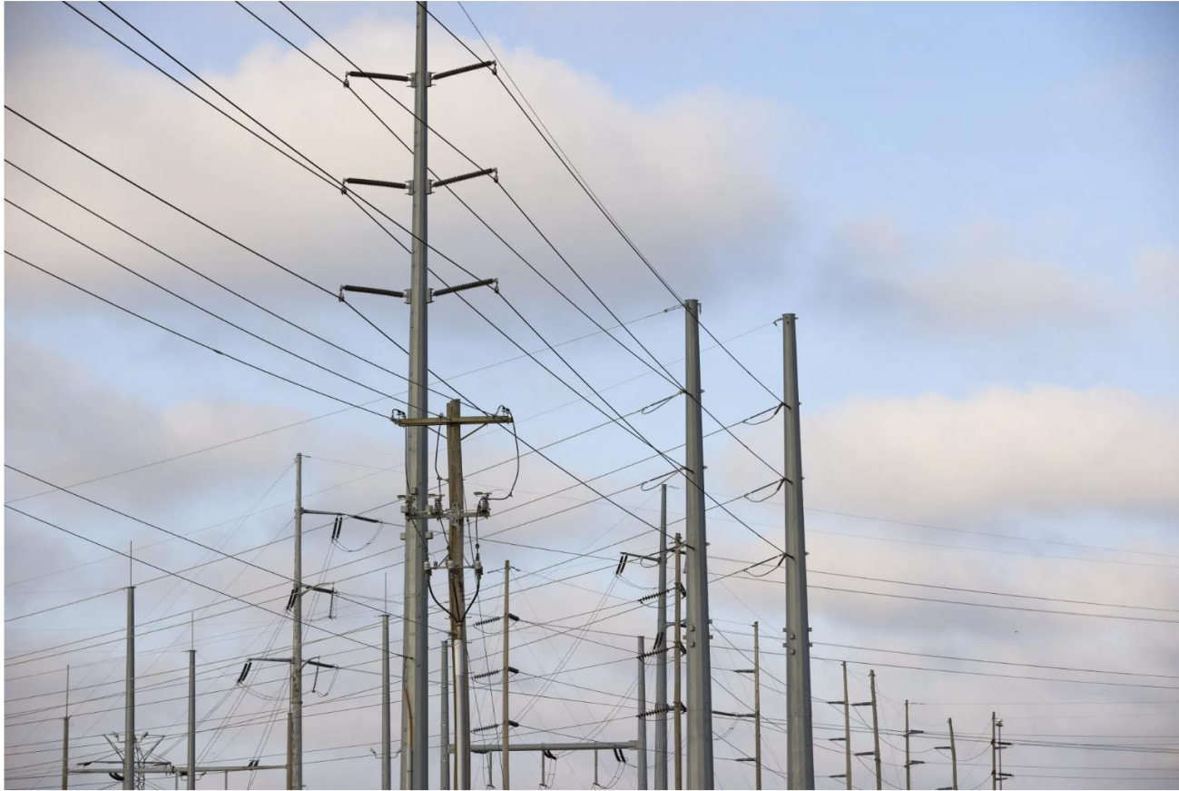
Transmission lines and electricity infrastructure adjacent to a data center in Hilliard, Ohio. Photographer: Brian Kaiser/Bloomberg
